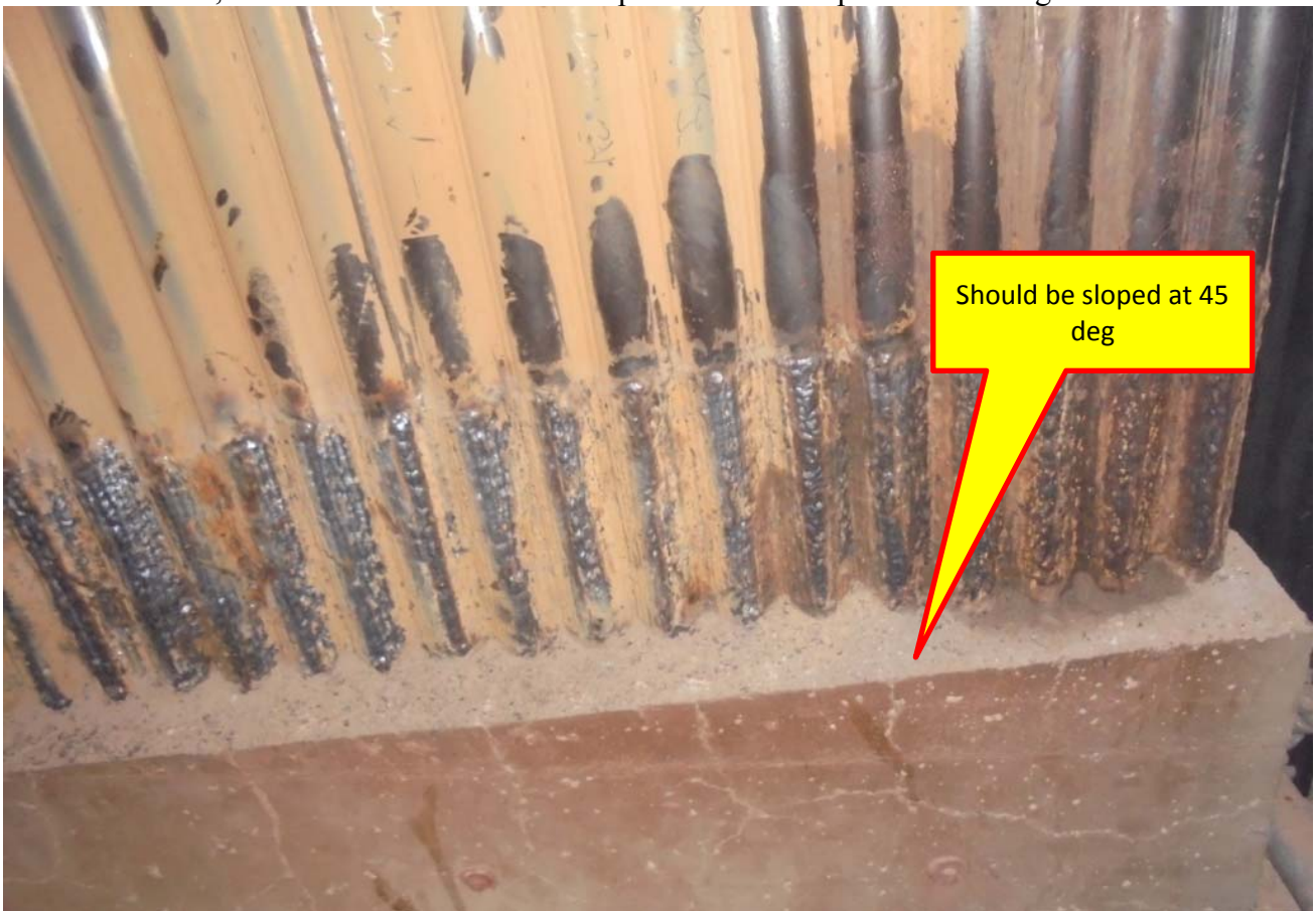
Photo 49: Photo shows the repair of weld overlay zone in wing wall SH. The mistake here is that the refractory should be sloped at 45 deg to allow free flow of solids without much resistance.
