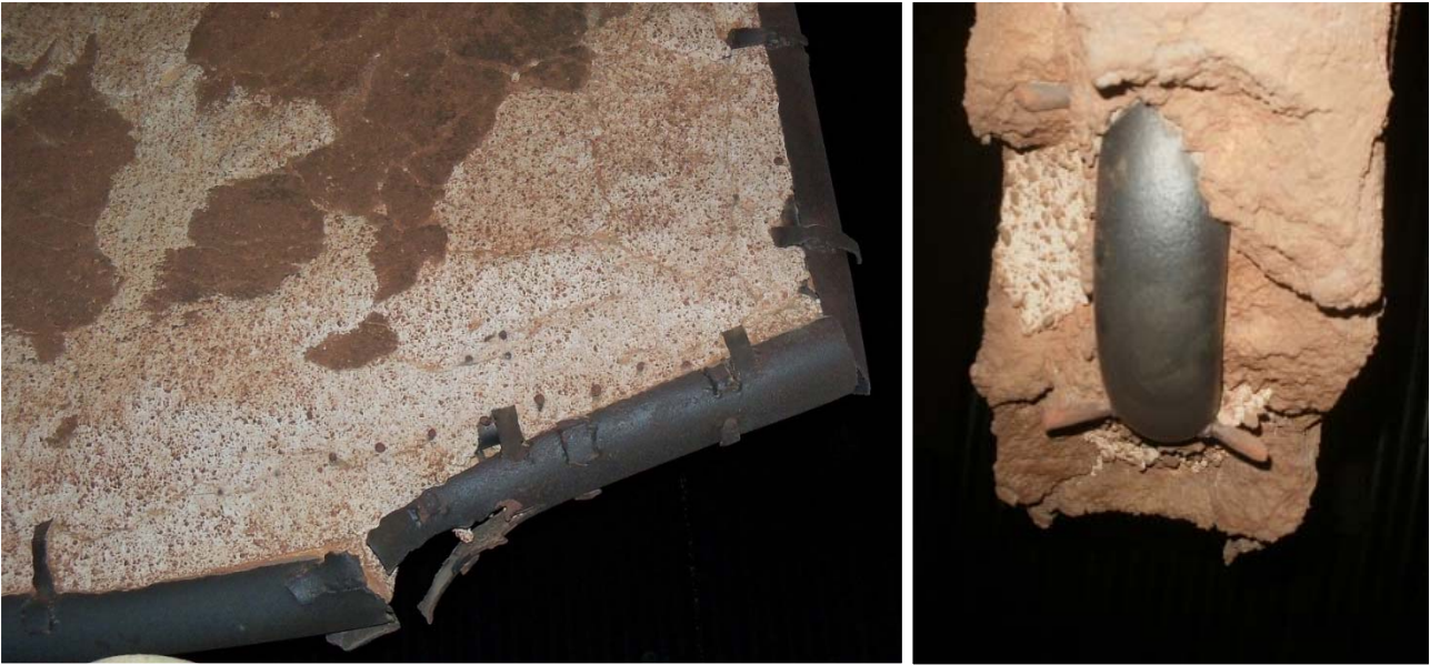
Photo 21 & 22: The above photos show poor practices by some boiler makers. Left side photo shows the inappropriate protection system. Right side photo shows the absence of studs to hold the refractory at the bends.
