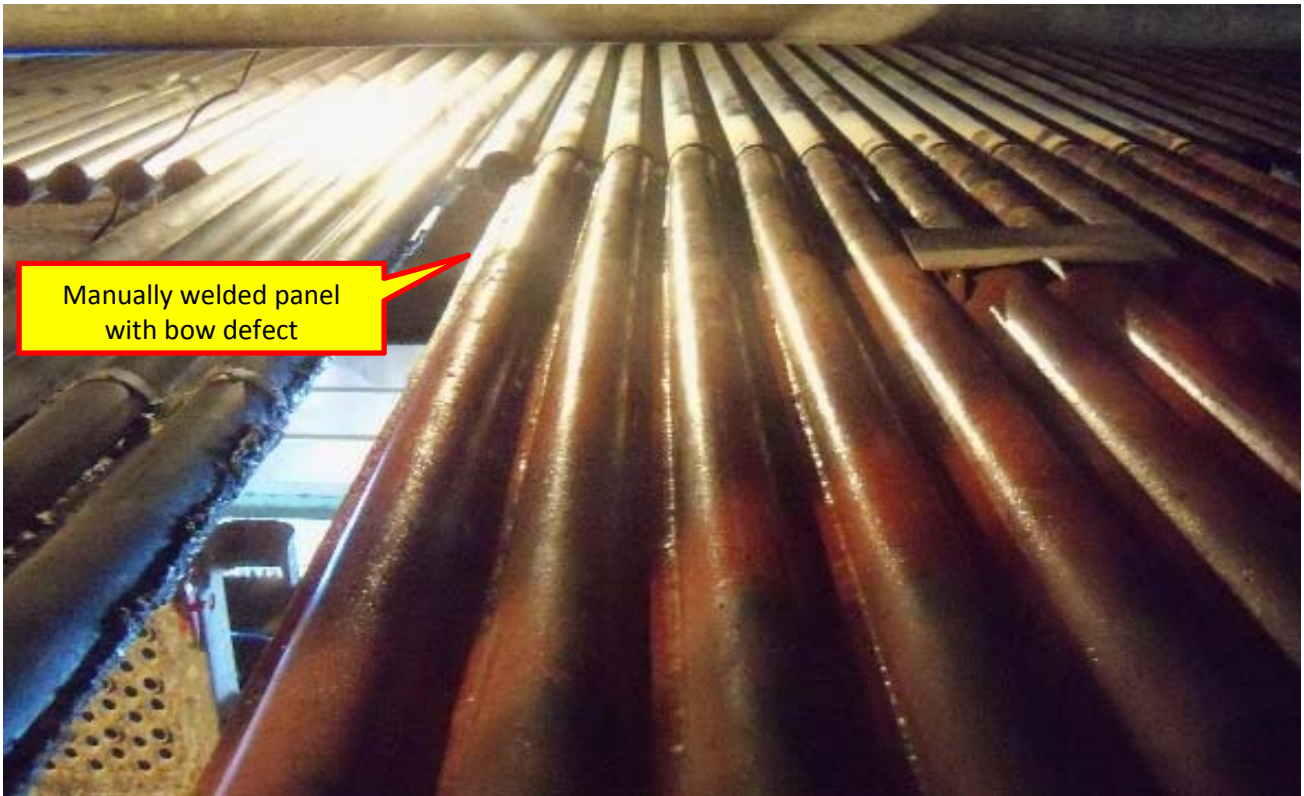
Photo 35: Photo shows the out of alignment of manually welded panel below the original machine welded panels. Boilers owners have to procure the spare panels only from parties who would deliver the panels duly welded in mechanized welding machine. Panel replacement team should be clear about the quality requirements at field.
