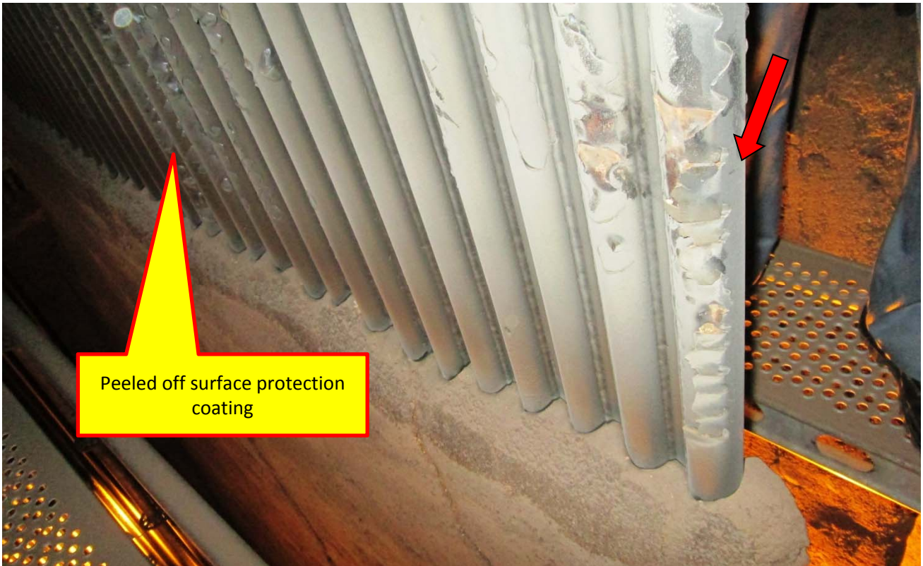
Photo 48: Photo shows the peeling of the HVOF spray over the wingwall evaporator panel. Field repair is not successful, unless it is executed with complete removal of previous coating.
