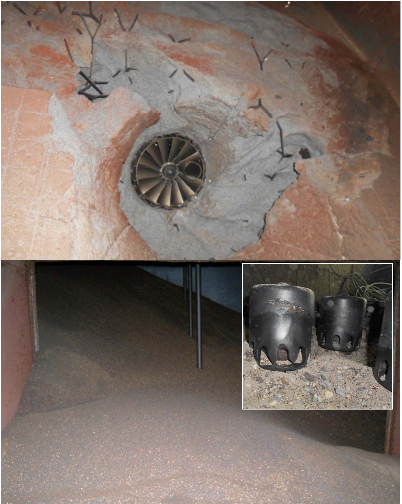
Photo 12 -14: Thick refractory in CFBC furnace walls is prone for spalling on account of thermal expansion. The air nozzles get eroded when the spalled refractory fall in between the nozzles and obstruct the air path as they get stuck near / at air nozzle openings. Air nozzle failures cause combustible bed material seepage in to the windbox. This is a serious hazard starting from simple refractory defects. Bottom photo shows the accumulation of bed material inside the windbox.
