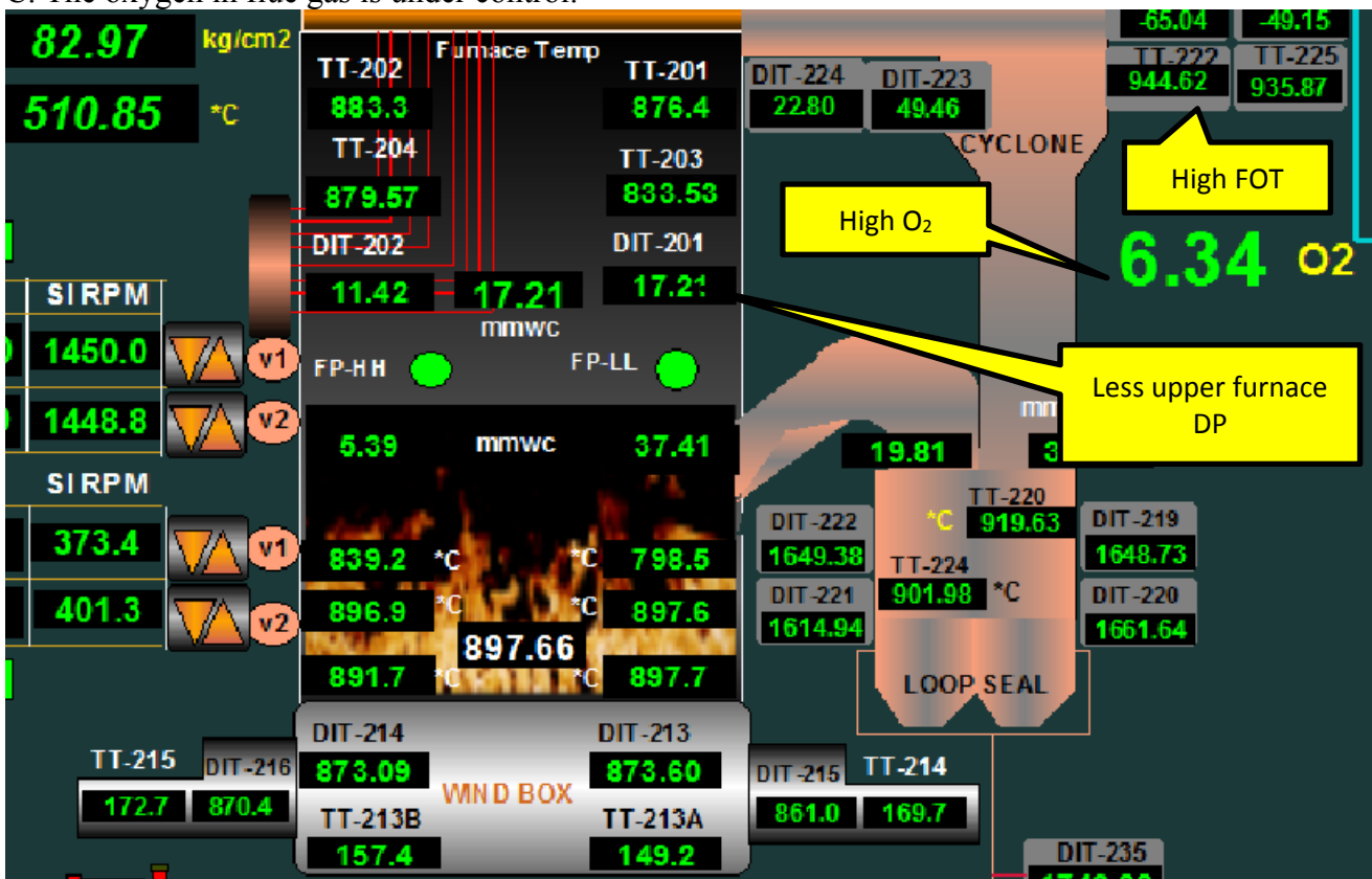
Photo 2: The upper furnace DP is hardly 17 mmWC. The cyclone outlet temperature is 936 & 945 deg C even with O 2 at 6.34%. The cyclone had not been performing well or the solids input from fuel had been less. It is net retention effect of addition, depletion of fine solids to furnace.
