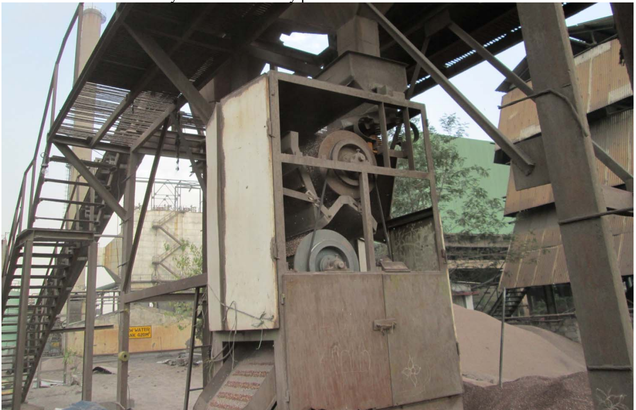
Photo 4: Drum type magnetic separator is used at plant to separate iron from bed ash. This will help to avoid rise in iron in solids inventory in the furnace. This is applicable for pyrite containing coals.
