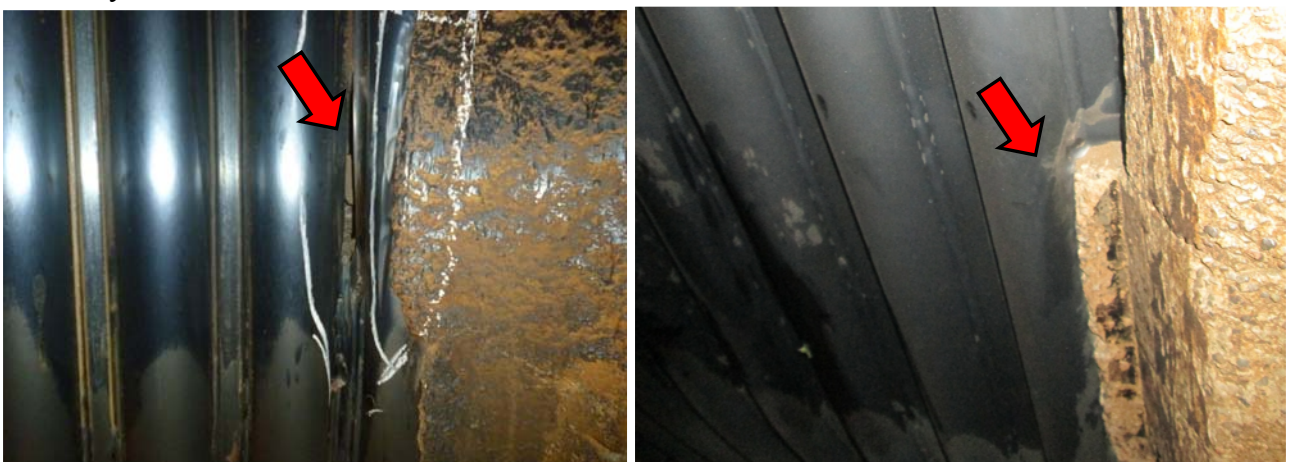
Photo 17 & 18: While the CFBC boiler demands a corner refractory detail for protection from erosion, improper design, improper application cause localized erosion. Localized deep cuts are seen in places of improper refractory tipping. Metal filling is to be done to stop the growth of the cut.
